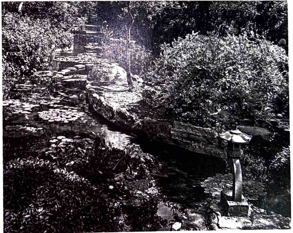
Lotus pond still filling after repairs and spray liner applied Photo by Bill Eger
