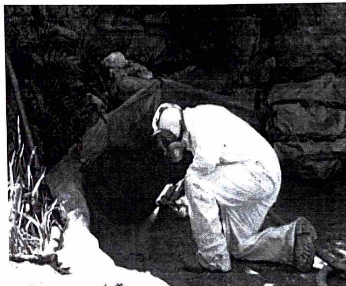
After carefully wrapping stones, pulling plants back, and masking edges by volunteers and park staff, the contractor finally had a dry day to apply the spray liner. Photo by Edward Parken for the Taniguchi Garden
